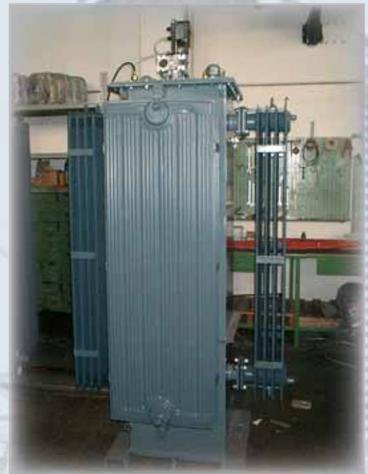
Voltage shield regulator
